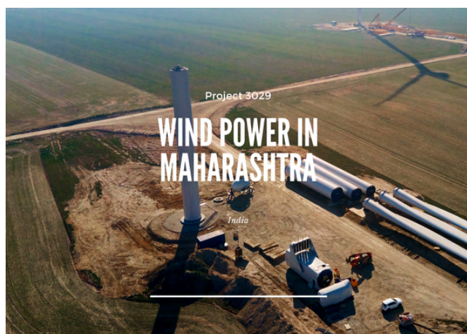
Project 3029: Wind Power in Maharashtra
